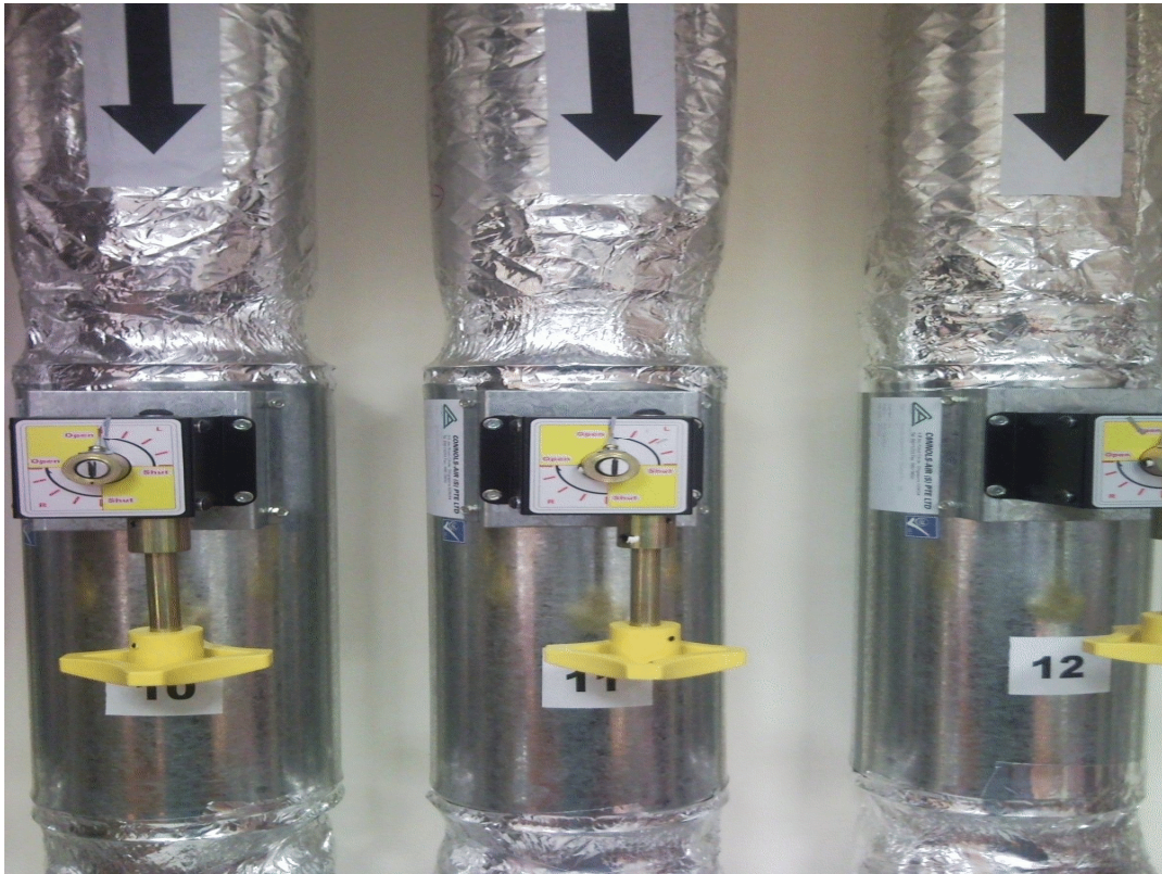
6.3 Manual damper to regulate airflow
